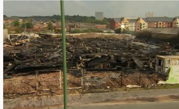
BBC, University of Nottingham laboratory fire caused by electrical fault, says report - BBC News
